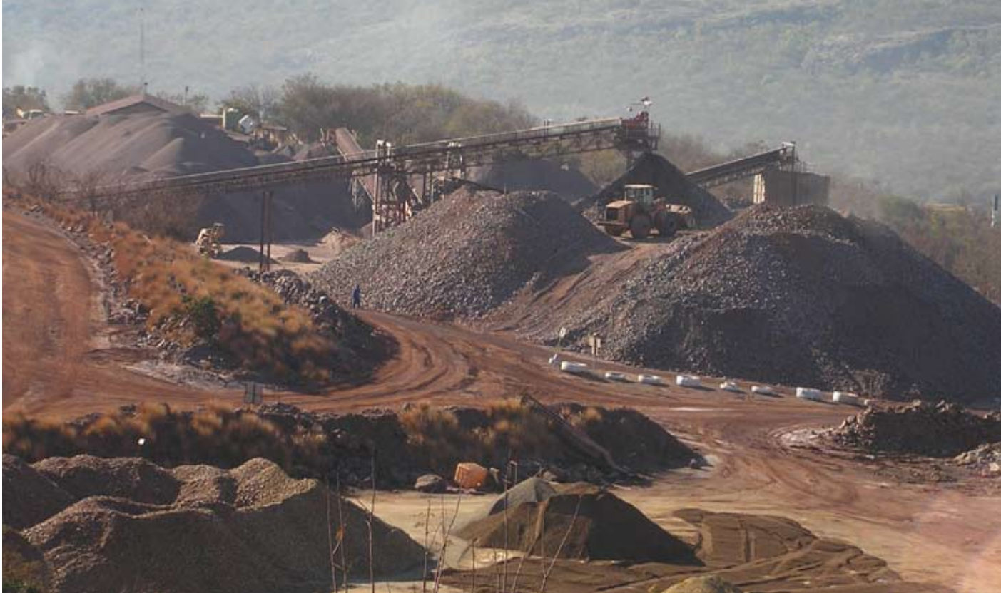
Primary stockpile and crushing facilities
